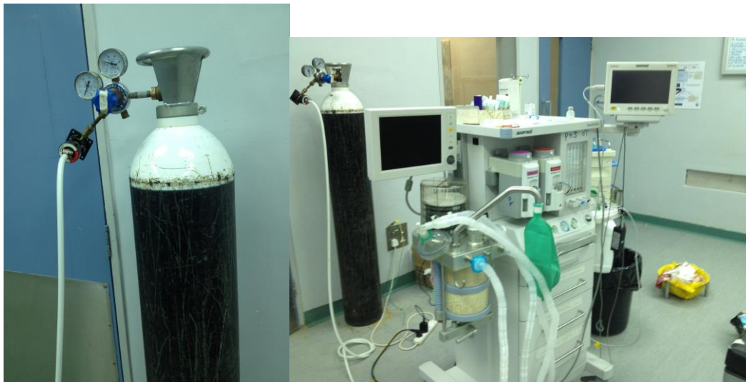
'Piped' Oxygen to anaesthetic machine, no other piped gases available
